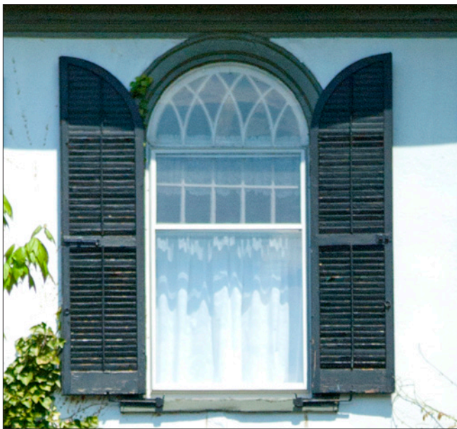
The blinds are sized and shaped to fit this half-round headed window. The storm window is also appropriate for the opening with horizontal rails aligning with the window elements beyond.
