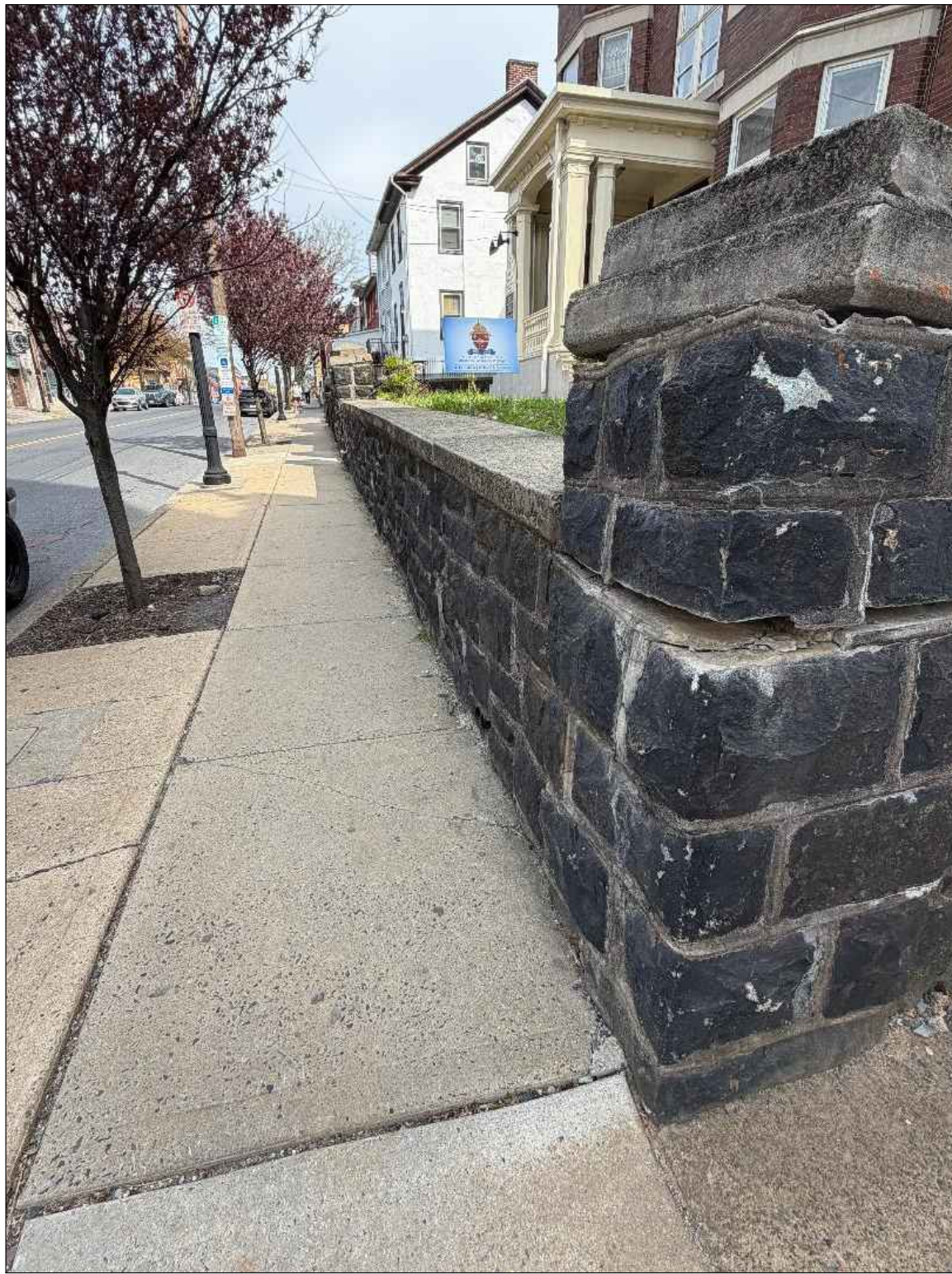
SHOWING TYPICAL DETERIORATION OF STONE WALL
