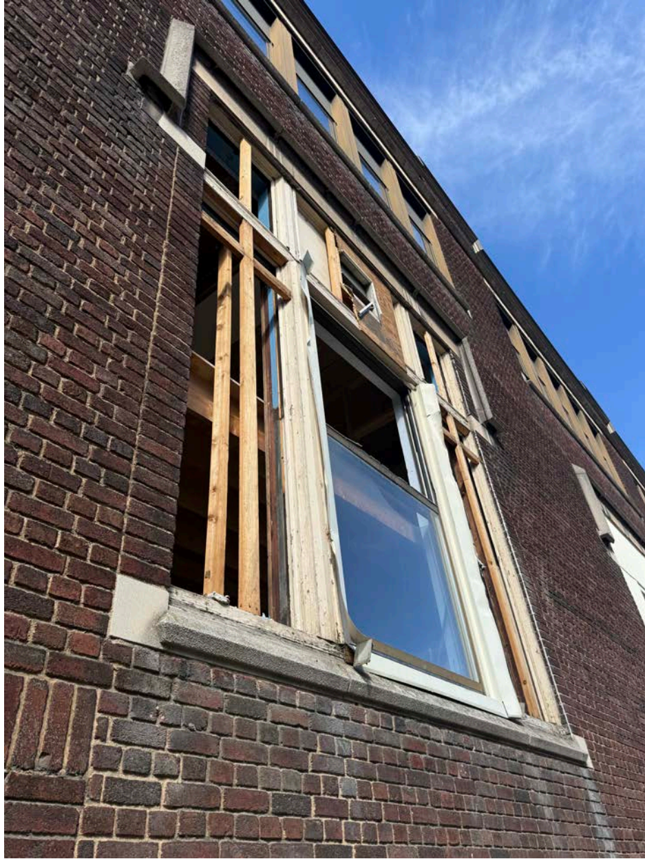
EAST FACADE - siding and plywood removed to reveal materials behind it. What was found was deteriorated wood and framing inside window openings that were used to install the plywood and siding.
