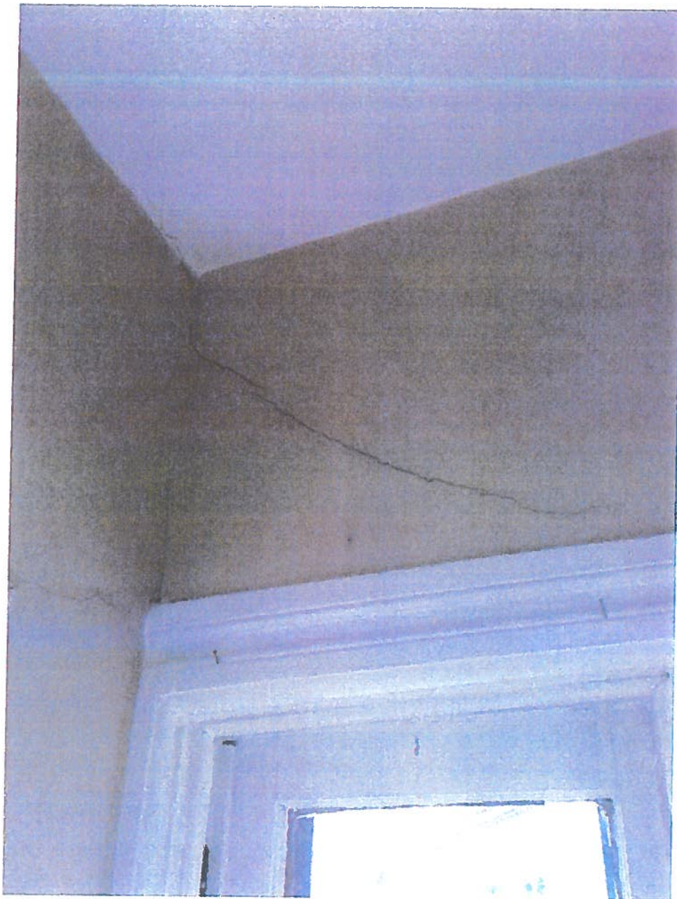
interior wall cracking
