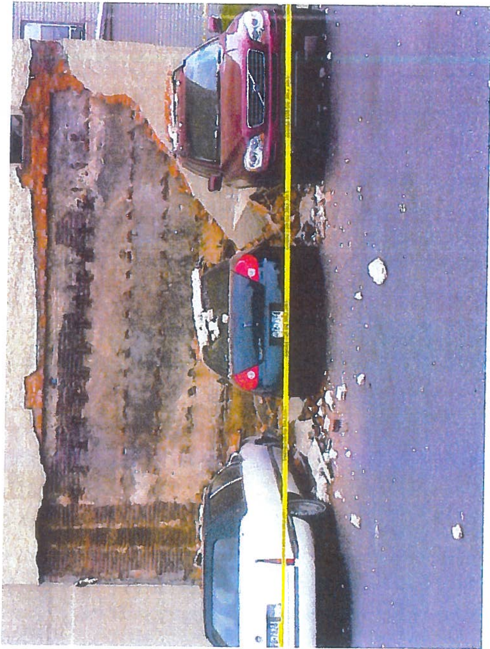
collapsed side wall
