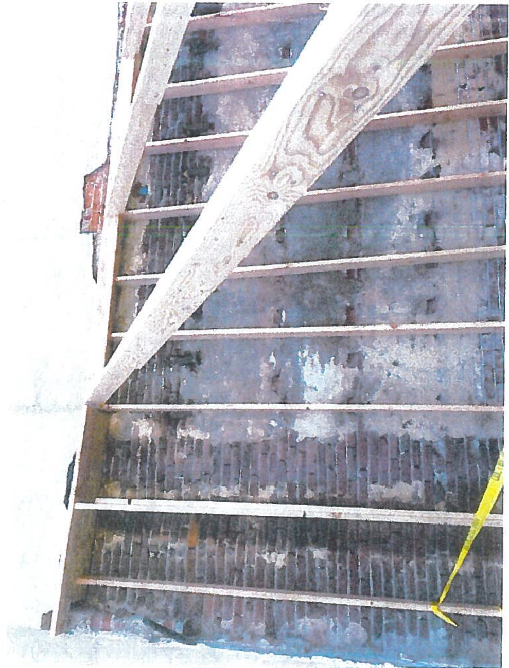
temporary support at collapsed wall
