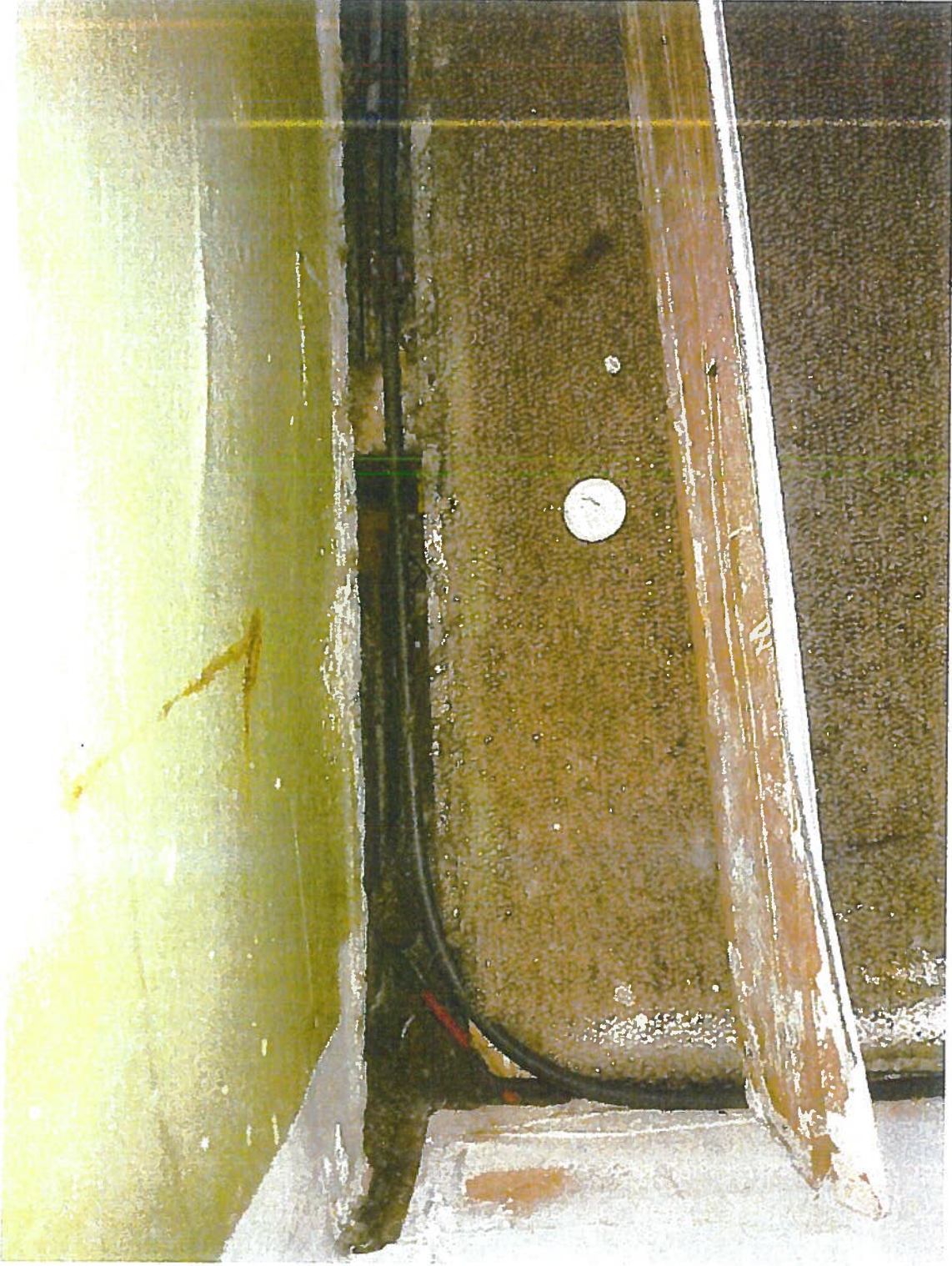
gap at wall/floor intersection
