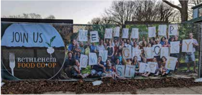
Pictured: A portion of the large banner spanning the construction site at 250 E. Broad St., future home of the Bethlehem Food Co-Op
