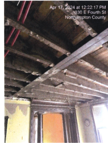
Exposed Joists in Ceiling of “Dining Room” – note also Steel Bearing Beam
