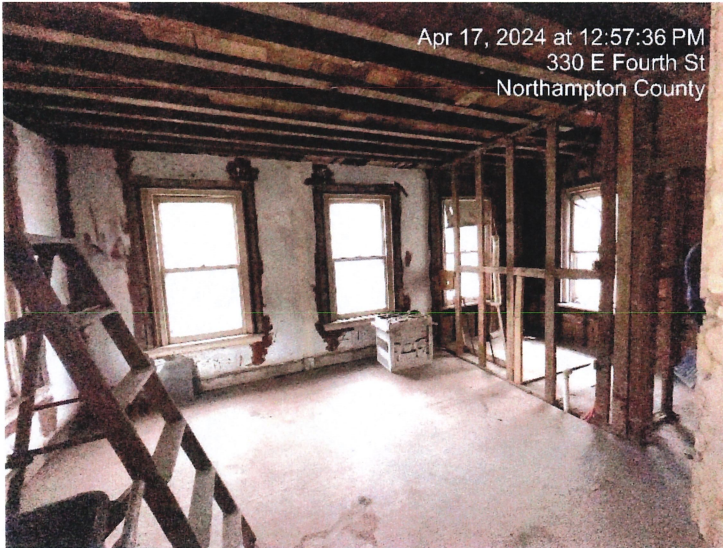
Back Room of 2nd Floor and Suspect Curtain Wall
