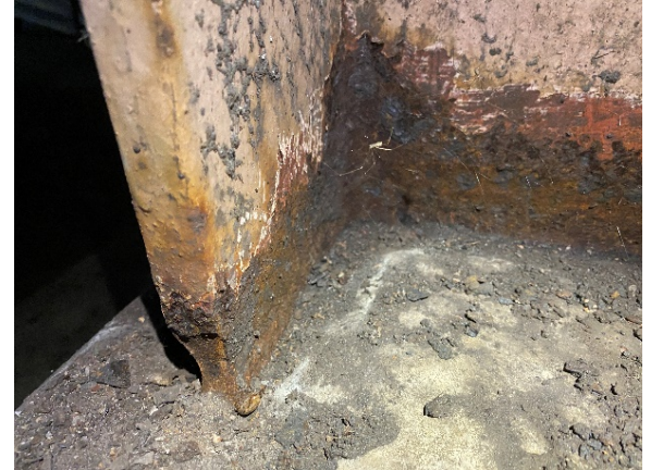
Deteriorating steel column
