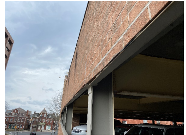
Broken welds at brick façade support
