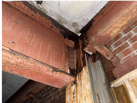
Example of deteriorating steel connection
