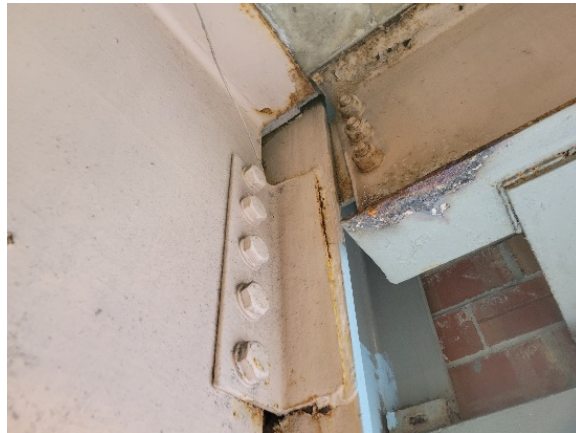
Failed Steel Connection (Cracked Welds)
