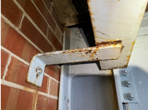
Failed Facade Connection (Cracked Welds)
