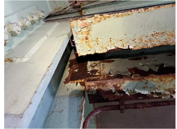
Deteriorating steel framing and connections
