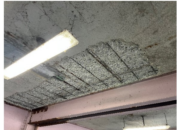
Deteriorating concrete deck
