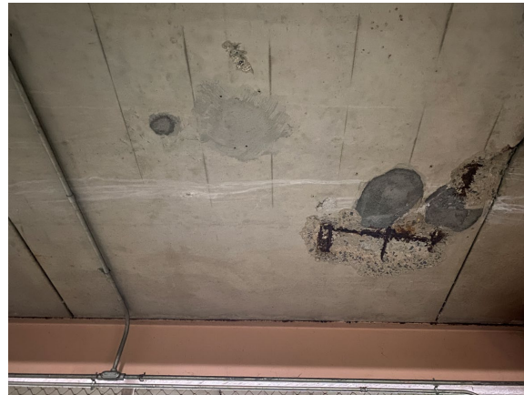
Broken prestress strands at ceiling of concrete slab
