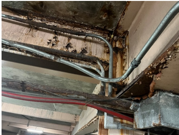
Deteriorating structural steel framing & connections
