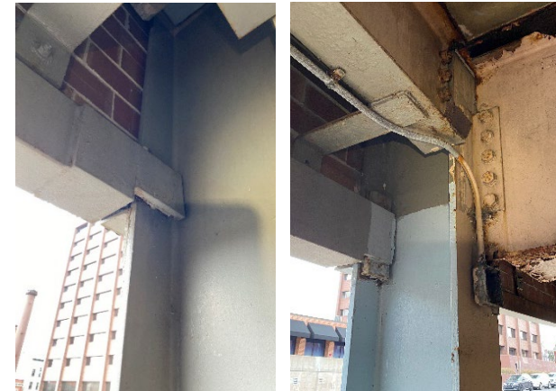
Broken welds at brick façade supports
