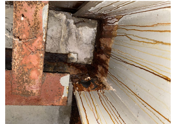
Example of deteriorating steel connection
