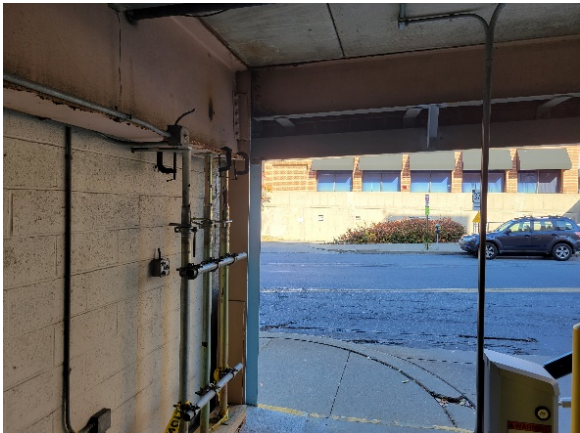
Shoring at Failed Steel Connection
