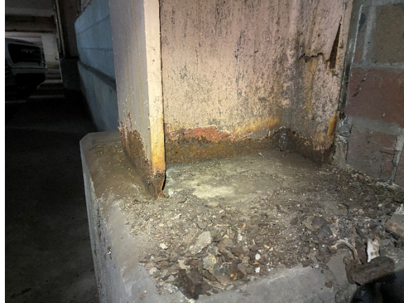
Deteriorating steel column
