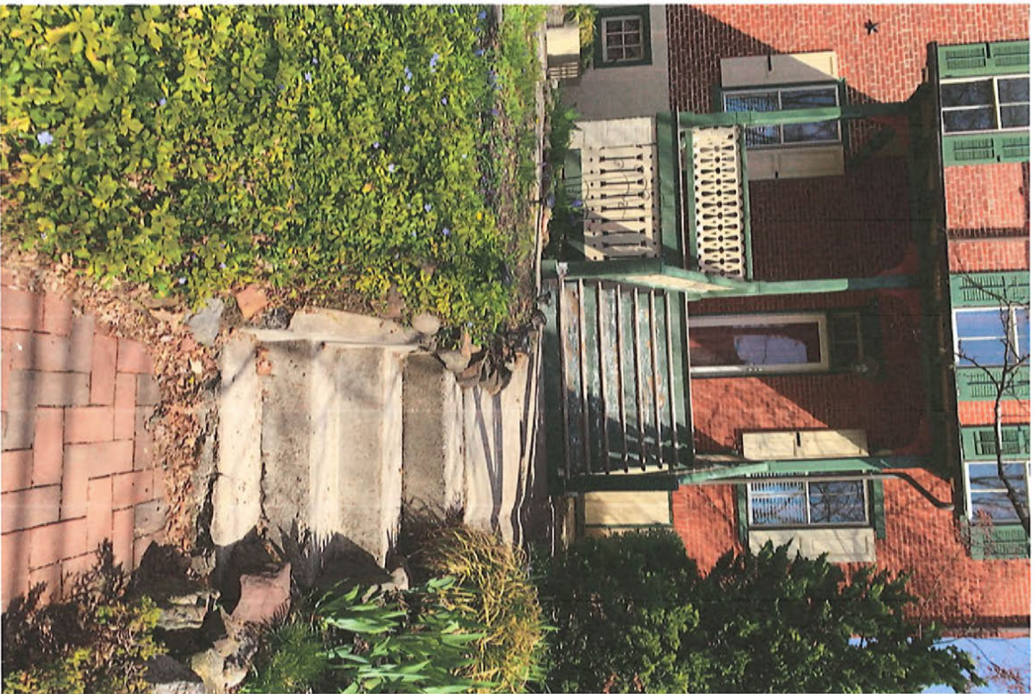
concrete stairs and landing to be replaced
