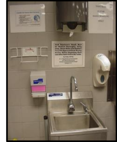
Handwashing sinks must be accessible at all times
