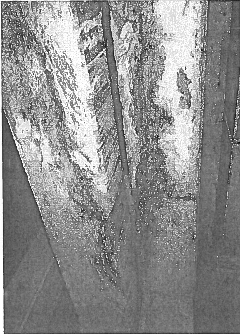
Photo 4: Item #2- Water infiltration due to failed expansion joint near the center of the plaza
