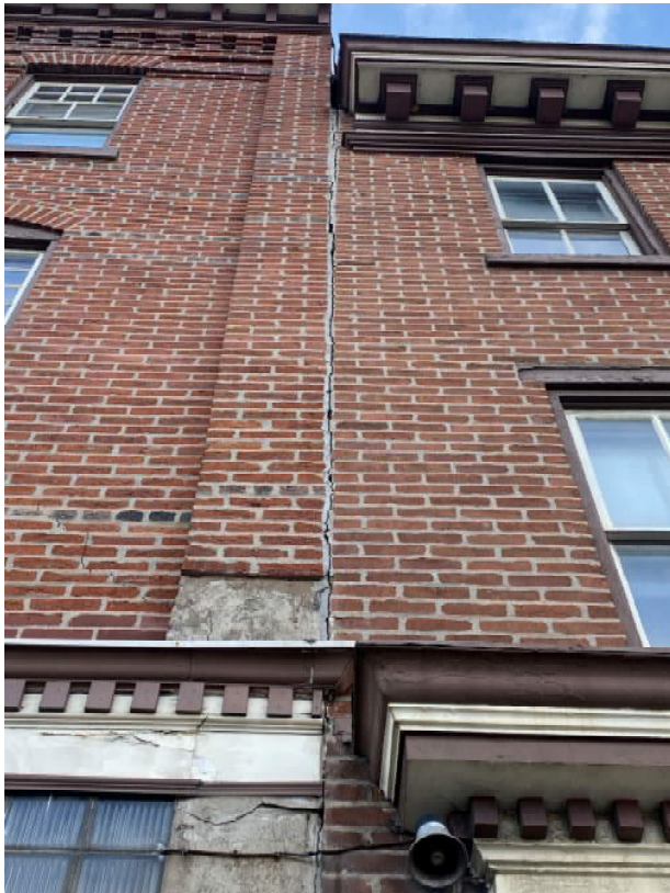
Photo 6 – Crack in north façade – widening toward the top.
