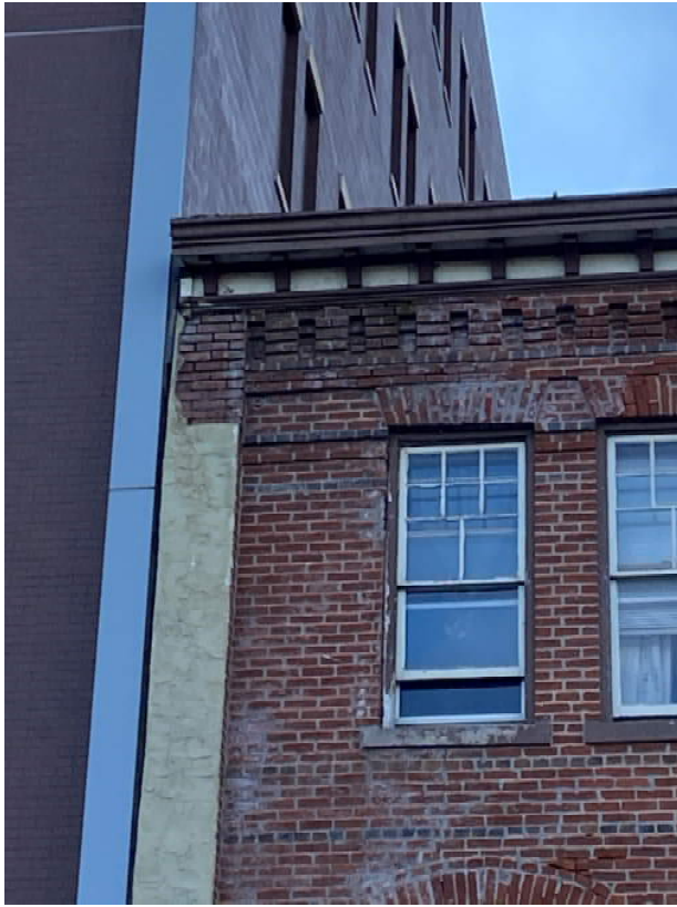
Photo 5 – Water infiltration on north facade
