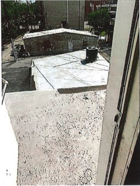
No egress on roof
