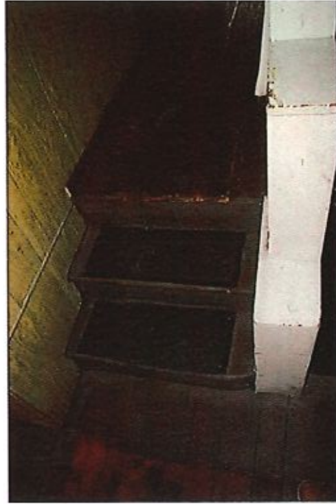
Unsafe split level stair
