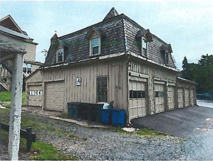
Adjacent Milton St. garage behind 30 E. Market St. Five of Eight doors are identical to door requested.
