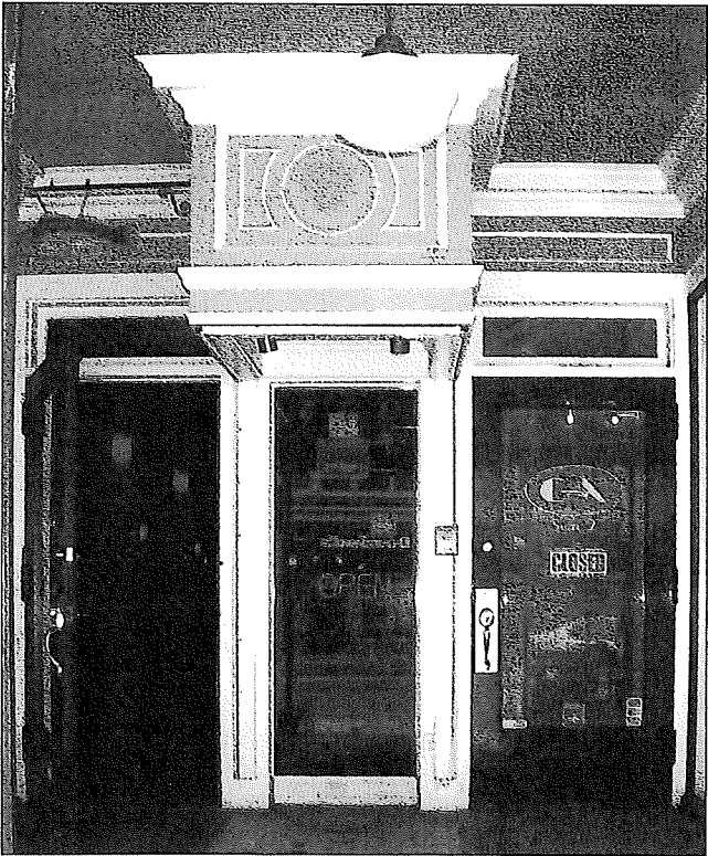
This pair of entrances located within the alcove provides access to the two businesses. The wood doors have large glazed areas that include applied signage and operable transom windows above.
