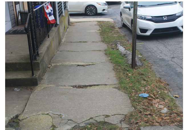
Residents are highly concerned about the lack of sidewalk maintenance, resulting in hazards for pedestrians.
