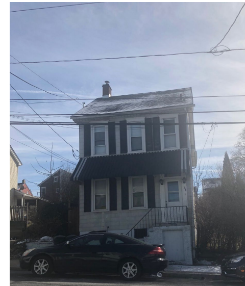
Figure 4: Some Market 2 homes had observable deferred maintenance related to roof or façade condition, but severe deterioration was rare.
