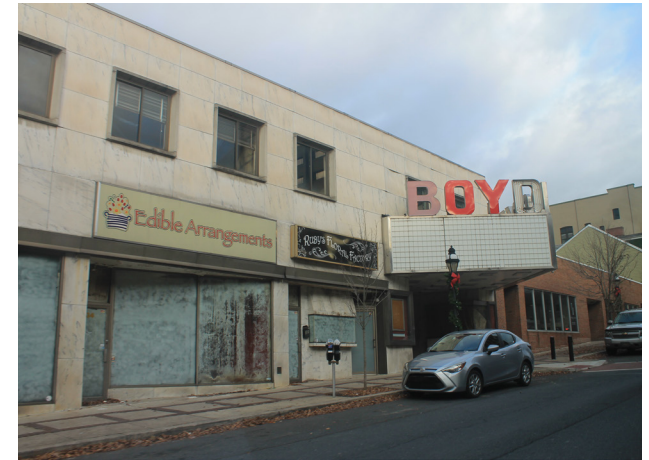
The former Boyd Theater building on Broad Street, which has been vacant and falling into disrepair for a few years.
