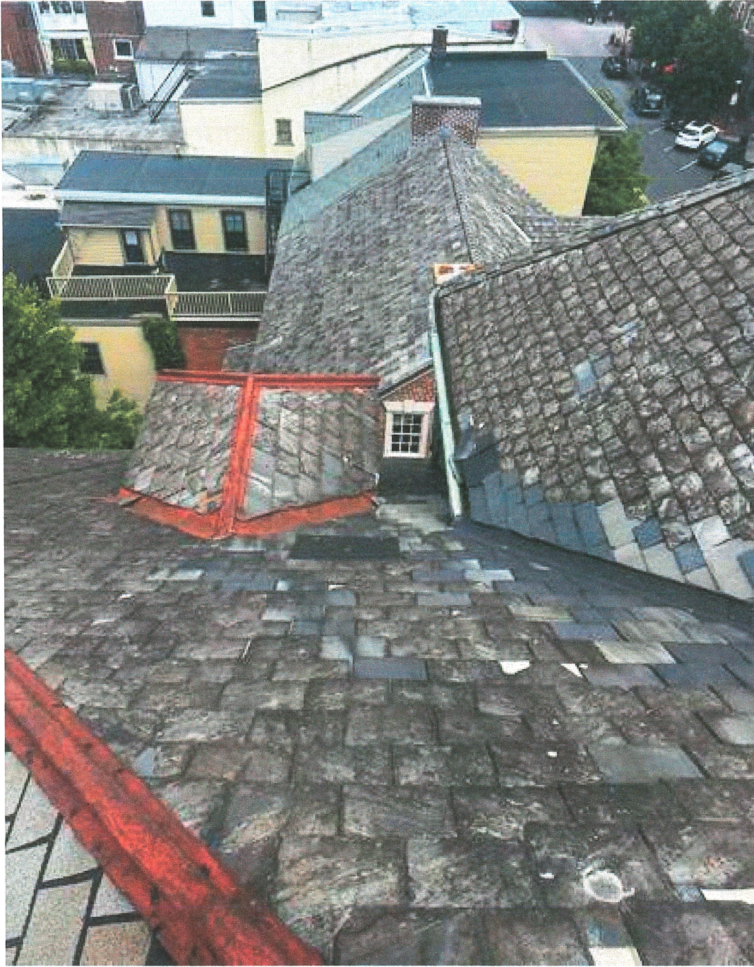
Slate tiles falling from roof due to nails backing out
