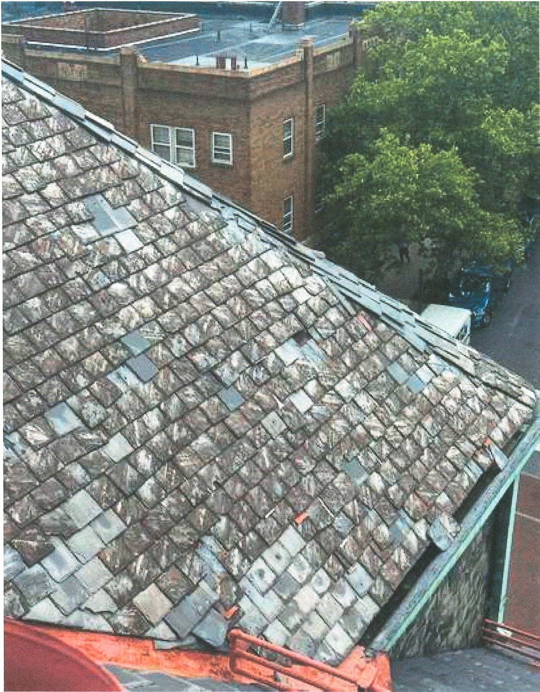
Loose slate tiles and severe de lamination
