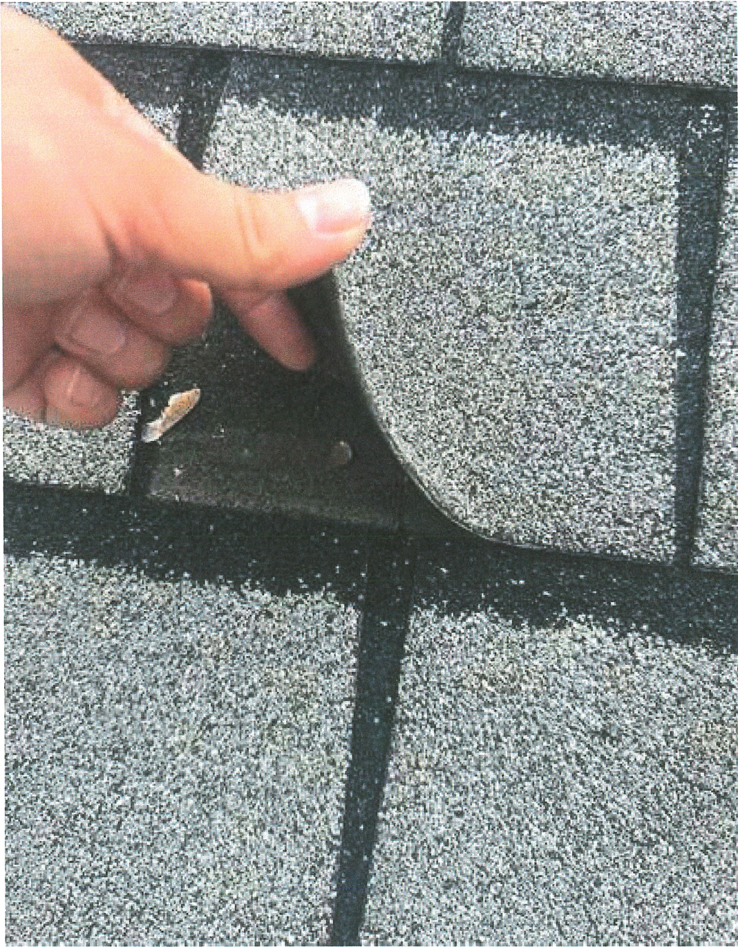
Nail backing out
