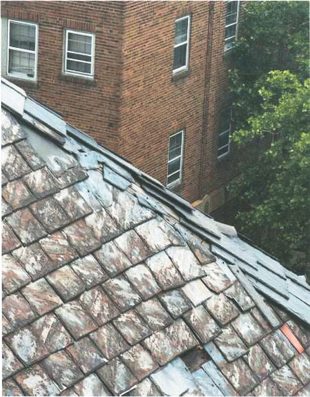
Loose Slate tiles
