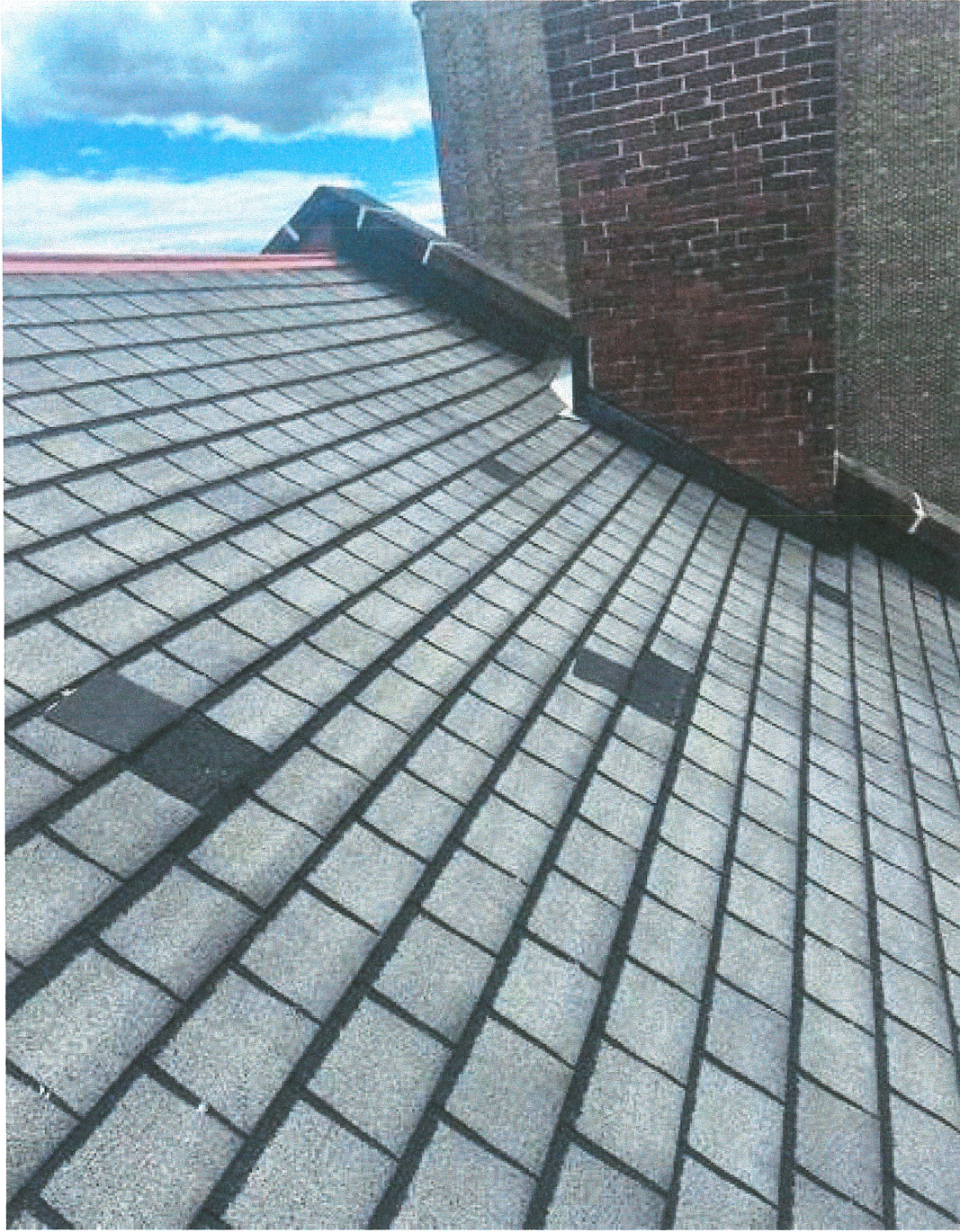
Shingle blow offs, needs new chimney flashing and step flashing around wall line.
