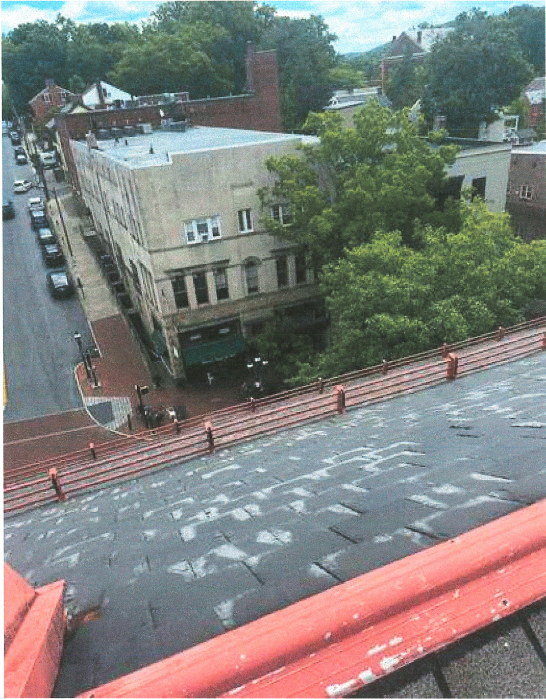
Flashing needs to be install around metal base frame
