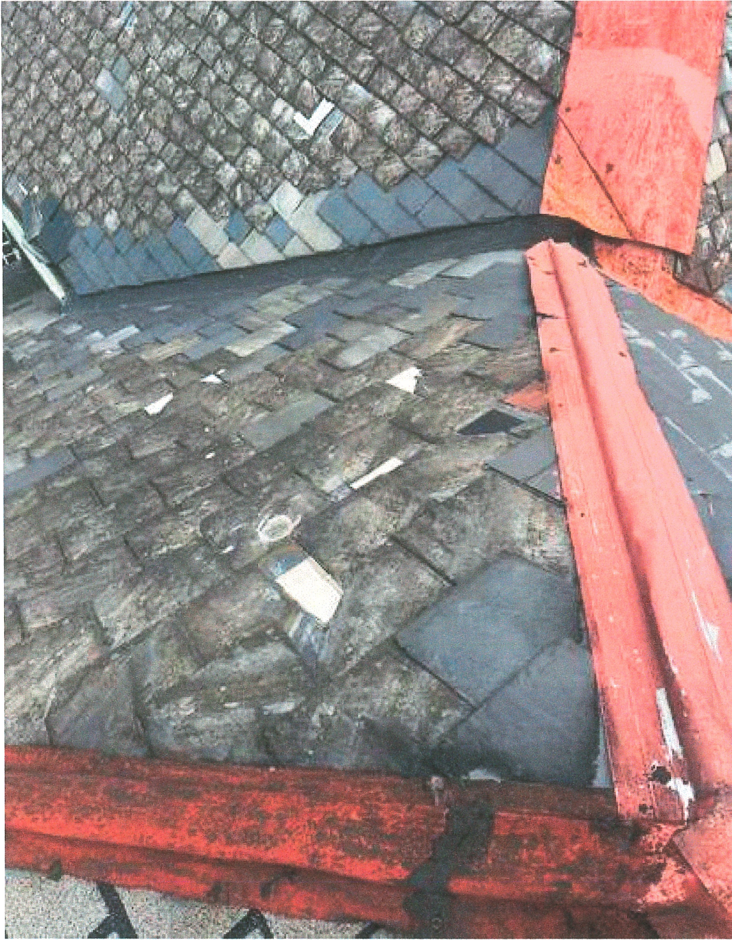
Roof was previously tried to be repaired unsuccessfully
