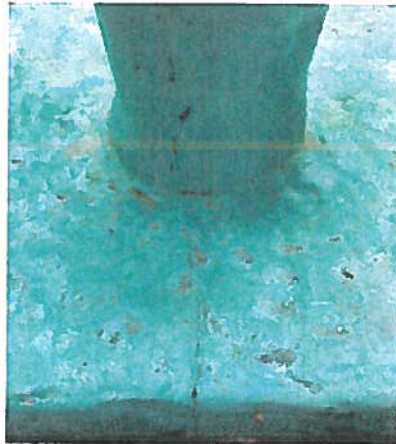
Further cracking on neck and base
