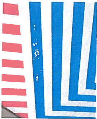
image showing paint loss and cracking
