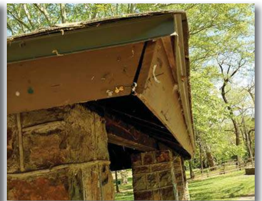
Pavilions #1 and #2: Damaged fascia boards.
