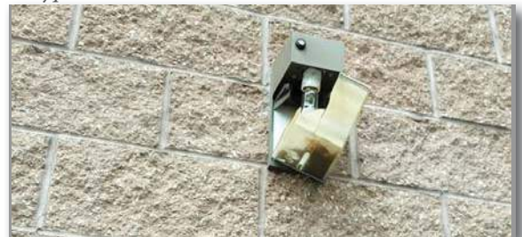
Damaged Light Fixture
