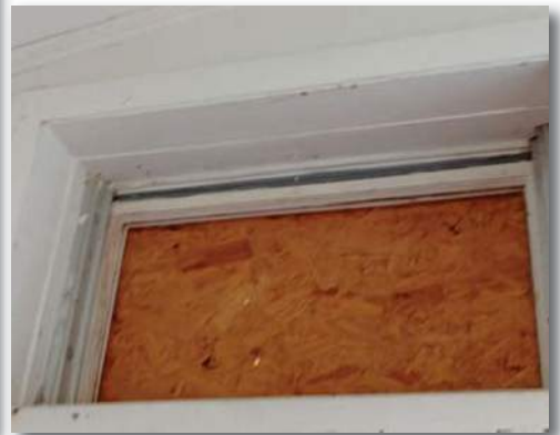
Several windows broken and boarded over.
