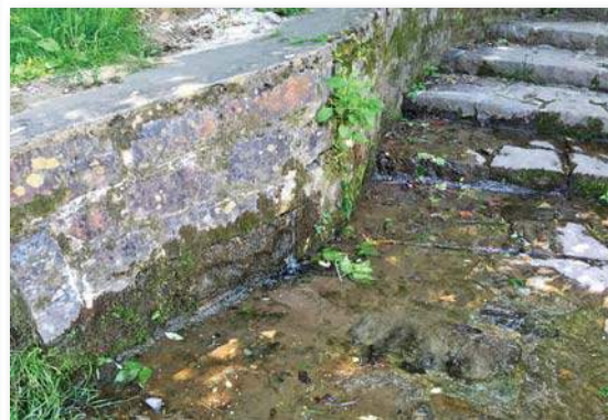
Leaking Wall near Dam
