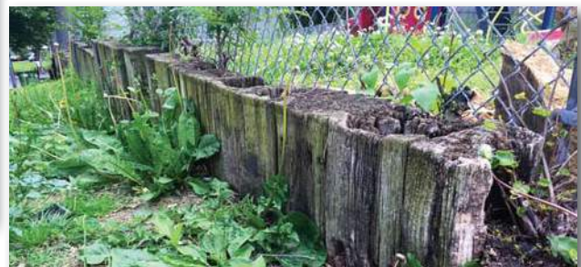
Timber walls support the park on two sides. These vertically installed walls are rotting.
