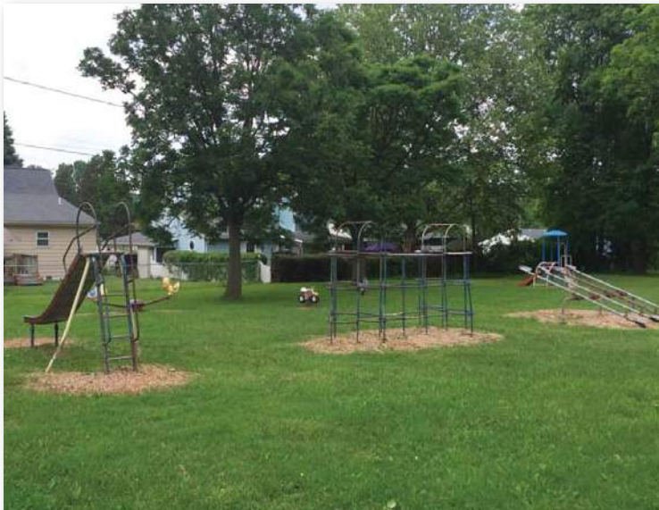
Play equipment is some of the most outdated in the city. Fall zones are inadequate. Peeling paint may contain lead.
