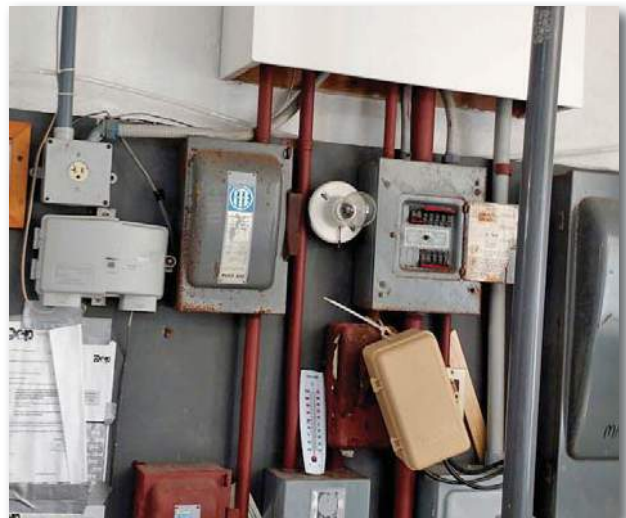
Electrical equipment over 30 years old. Manufacturer has history of product failure.
