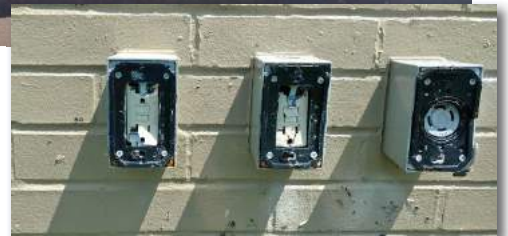
Unsafe, damaged exterior outlets.
