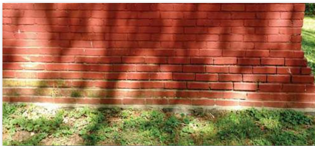
Deteriorating brick pointing typical at foundation.
