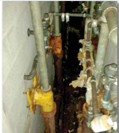
Pipe chase has leaking piping and pooling water.
