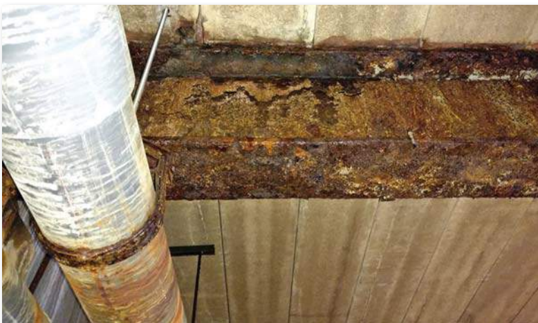
Deteriorating structural steel. The bearing points also show signs of degradation and cracking concrete.
