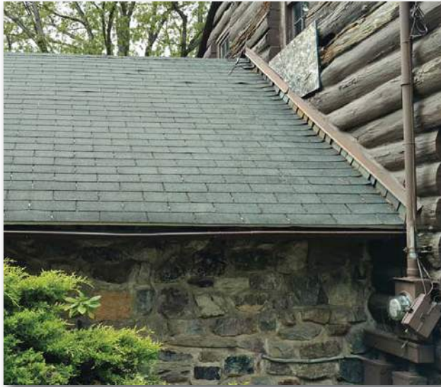
Damaged shingles, worn roof edge, deteriorating gutter and straps, facade and structure.
