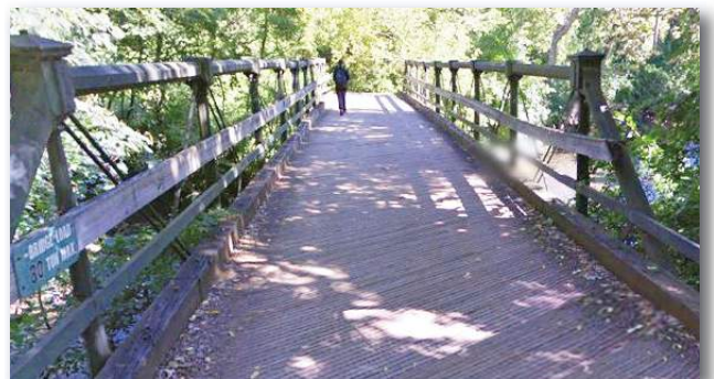
Wooden bridge crossing Monocacy Creek to D&L trail from Sand Island used by cyclists and pedestrians.
