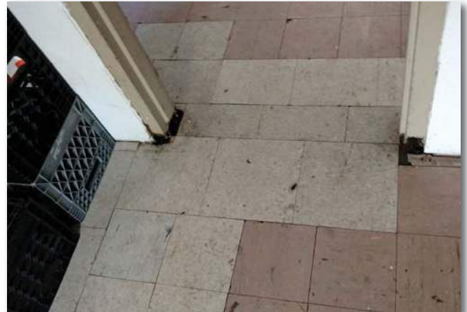
Damaged and mismatched floor tiles. Uneven surface and peeling tile presents tripping hazard. Rusted and rotted doors and frames.
