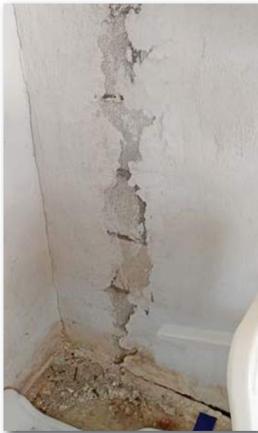
Cracks and delaminating finishes due to water infiltration.
