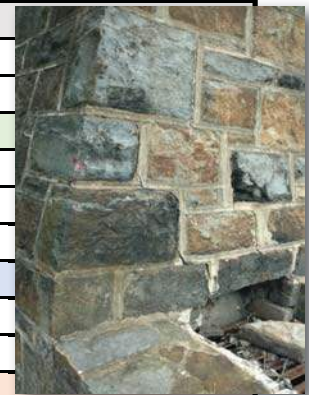
Cracks in masonry.
