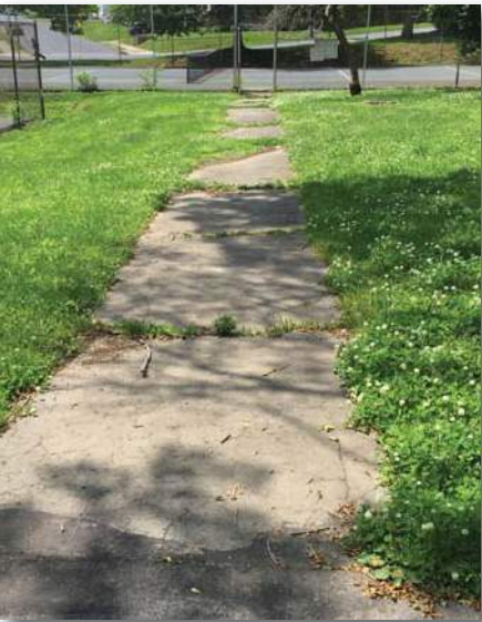
Paved path to tennis court, not ADA compliant. Condition Typical.
