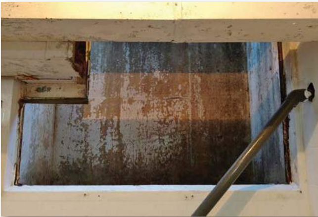
Open unenclosed light well. Bottom of well is full of leaves and garbage.
