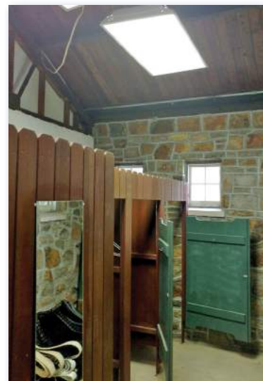
Non-ADA compliant toilet rooms.
