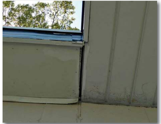
Building #2: Damaged soffit.
