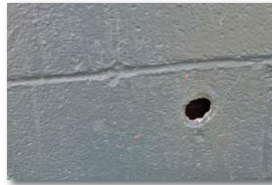
Building #1: Holes in CMU.
