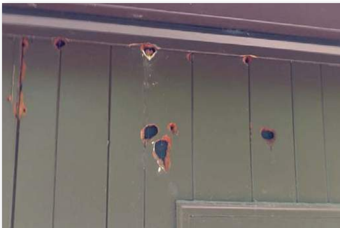
Toilet Facility: Holes in wood siding, insect and rodent damage.
