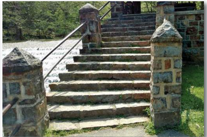
-Monocacy Creek Overlook Pavilion #3: Stone work has degraded pointing. No ADA access.
