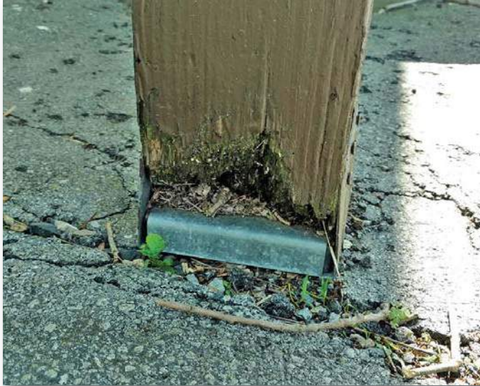
Rotted wood columns, typical throughout.
