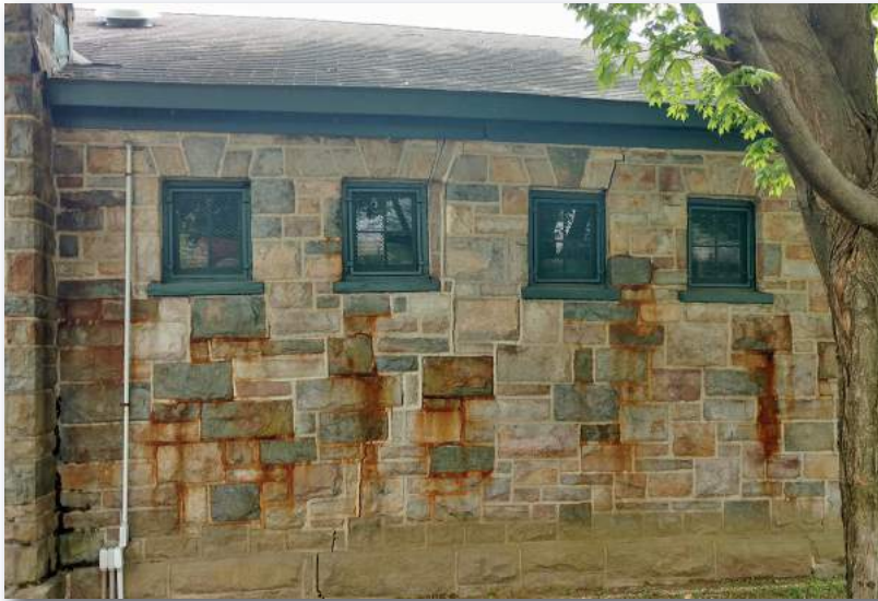
Right side of photograph: signs of foundation settlement. Large long cracks, roof buckling, and leaning building components.
