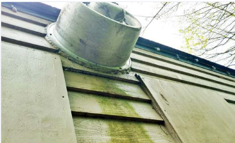
Exhaust fan shows sign of leaks and rotted siding.
