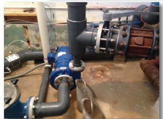
Corroded Flow Control and Valving
