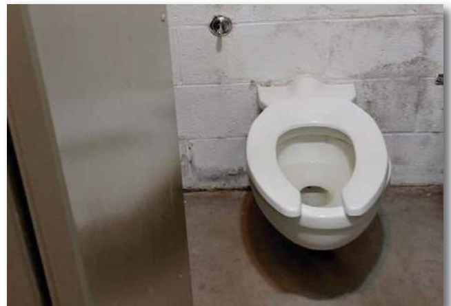
Toilet Facility: Non-ADA compliant toilet rooms.
