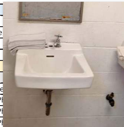
Non-ADA complaint toilet room fixtures, no insulated protectors, missing mirrors.
