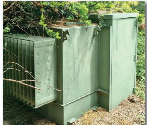
Over grown plantings around electrical transformer.
