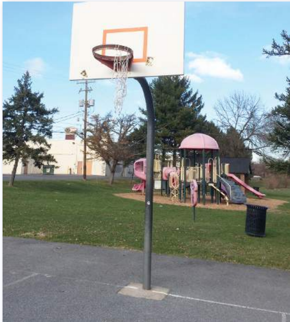
Basketball nets in poor condition. Faded lines on courts.
