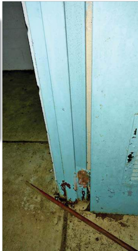
Rusted and Deteriorated doors & frames
