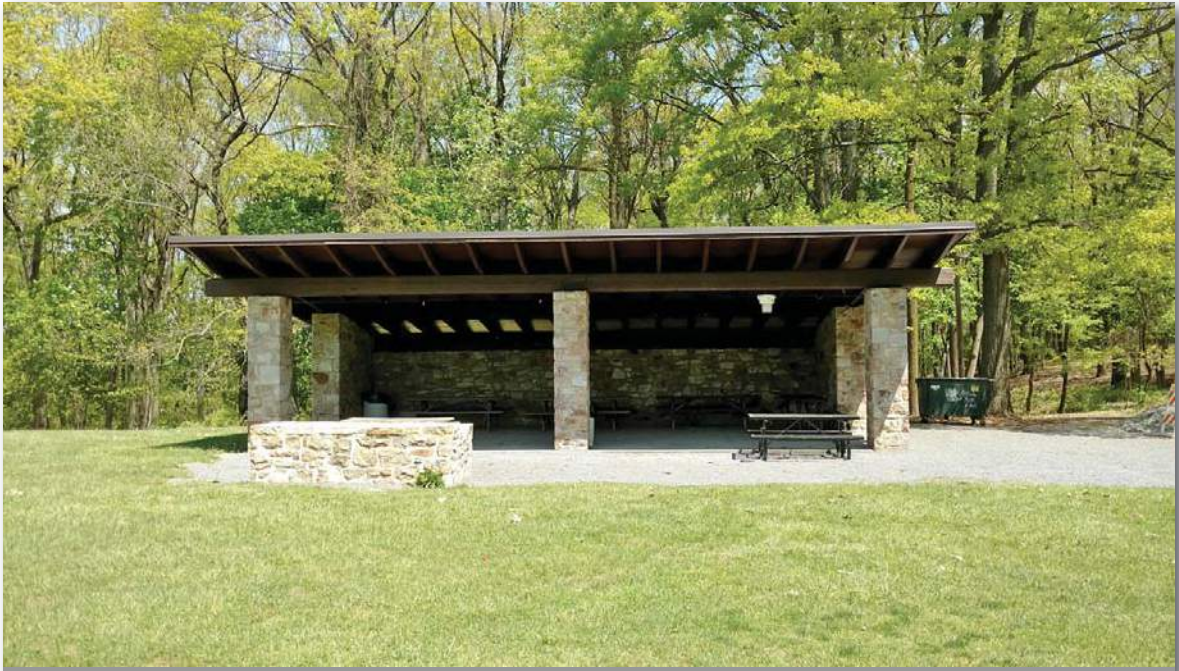
Pavilion#2: Missing mortar joints, areas of insect damaged or rotted fascia.
