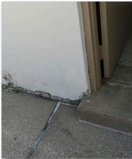
Degraded foundation and non-ADA compliant entry way.
