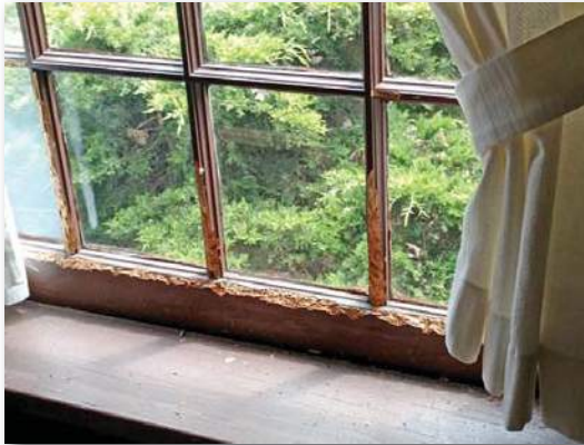
Animal damage on window sash.
