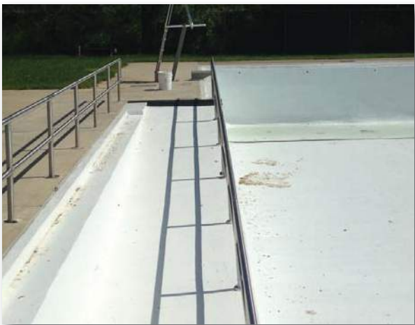
ADA Ramp does not meet current criteria
