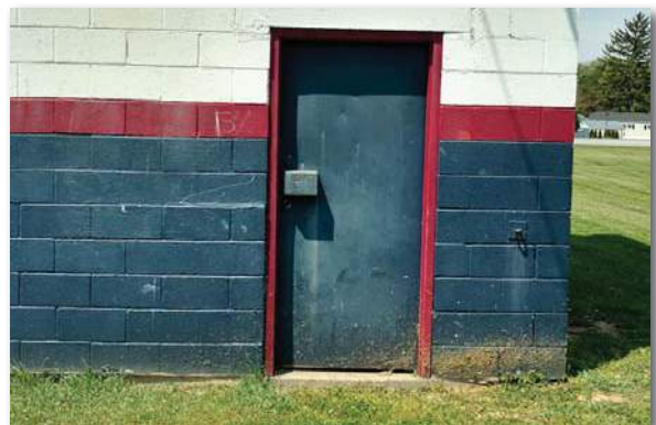
Building #1: Damaged door.
