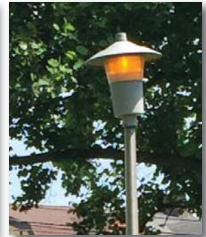
Dated Light Fixture not efficient and damaged
