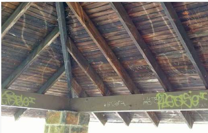
Monocacy Creek Overlook Pavilion #4: Graffiti typical. Damaged or rotted roof edge typical.
