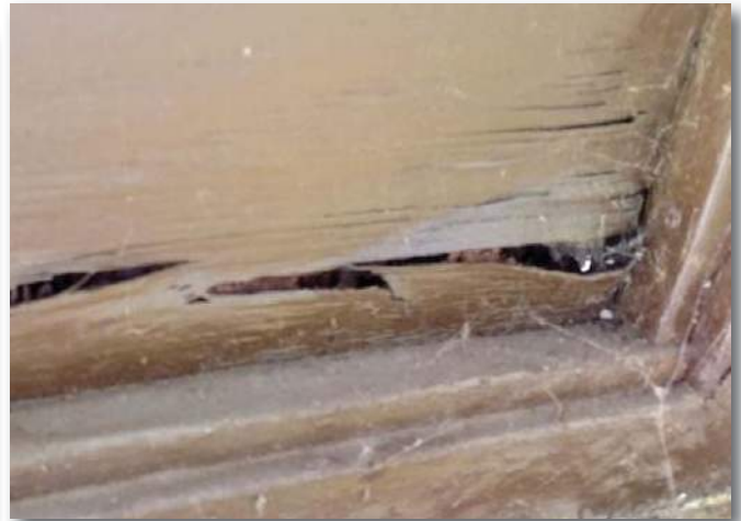
Rotting in-filled transaction window.
