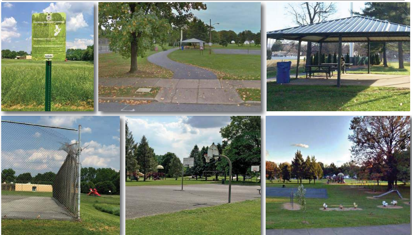
This park is typical of Bethlehem Parks, not well maintained. Some attention given to mulch , but fall zones are inadequate and there is no ADA access to facilities in the park. The courts are in fair condition, lines faded, not coated, tennis court fencing damaged and rusted. No mow meadow reduces mowing and separates park from school property.
