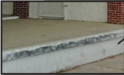
Damaged and chipped concrete edge.
