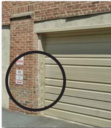
Damaged and dented frame.
