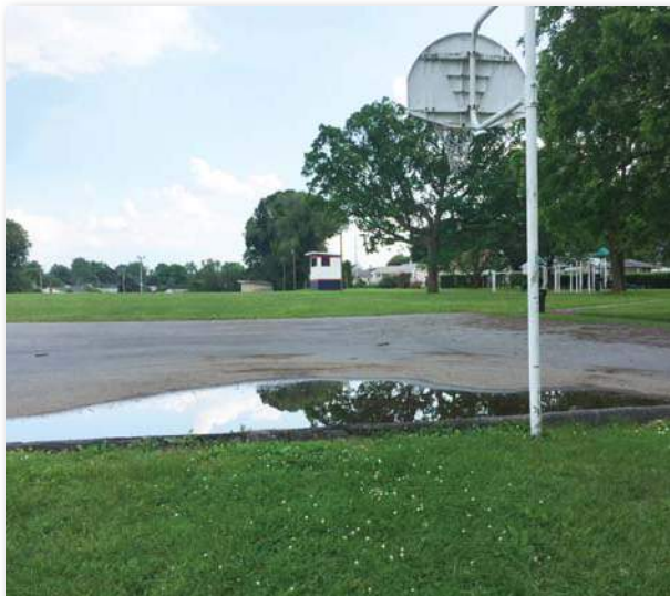
Basketball Courts in Poor Condition.
