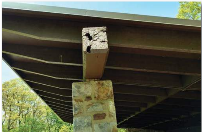
Pavilion#2: Rotting support beam, typical at each end.
