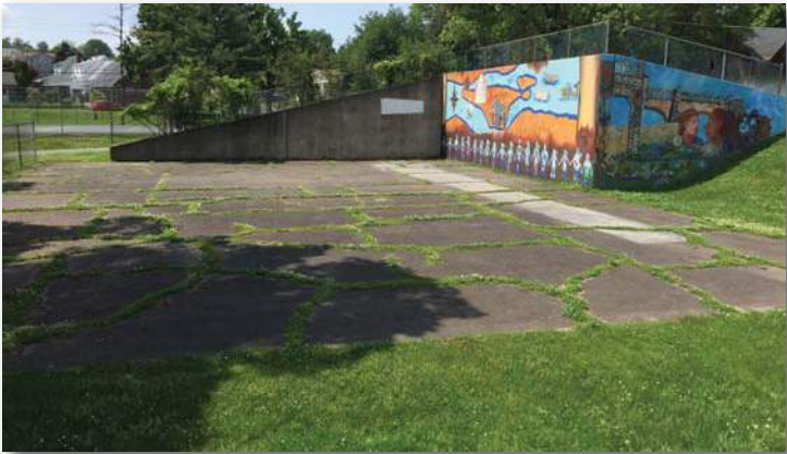
Unmarked area of pavement with mural wall surround. Pavement in poor condition, typical of paved surfaces throughout this park.
