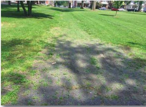
Gravel Pathway through park encroached by lawn grass. Not ADA compliant.
