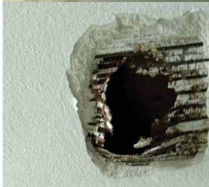
Signs of water damage, delaminating finishes and holes in ceilings.
