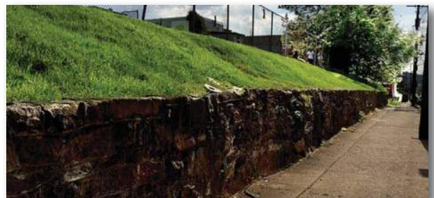
5.0' stone wall borders park on Third St., with no steps or way up. Residents access park from adjoining property on Third Street.
