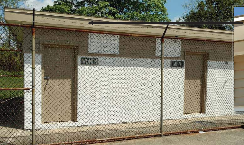
Degraded soffit and fascia board.
