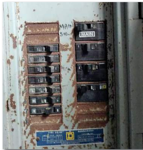
Electrical panel shows signs of corrosion.
