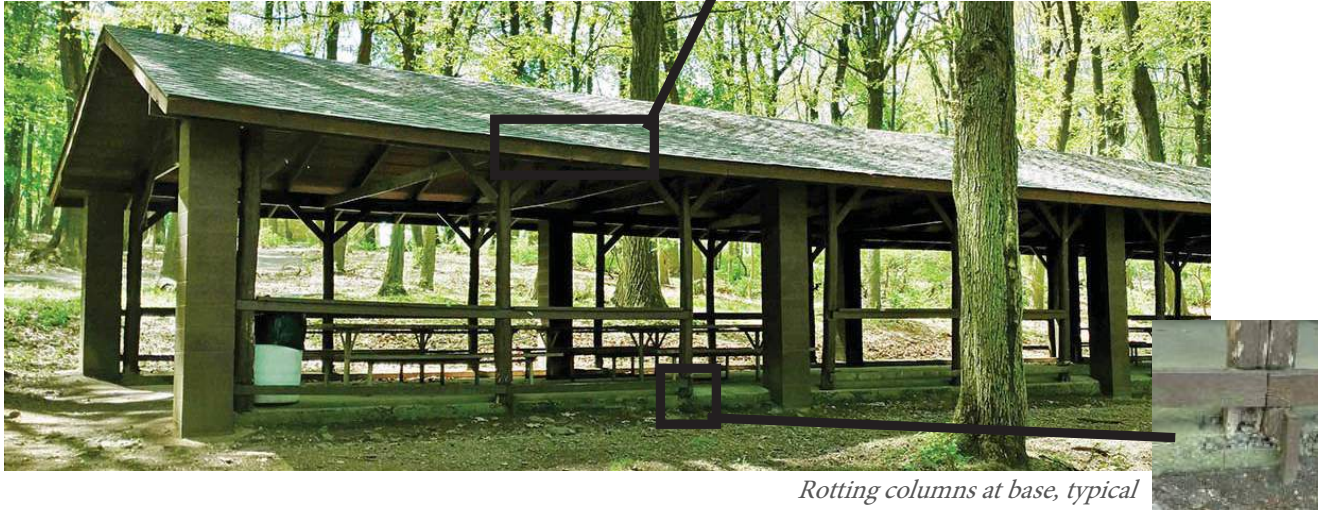
Broken and rotted fascia board, typical
