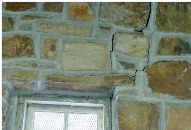
Cracks in masonry and patched pointing.
