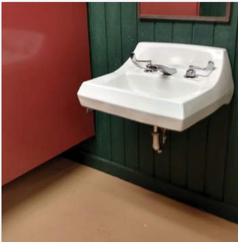
Missing ADA insulated covers for sink piping.
