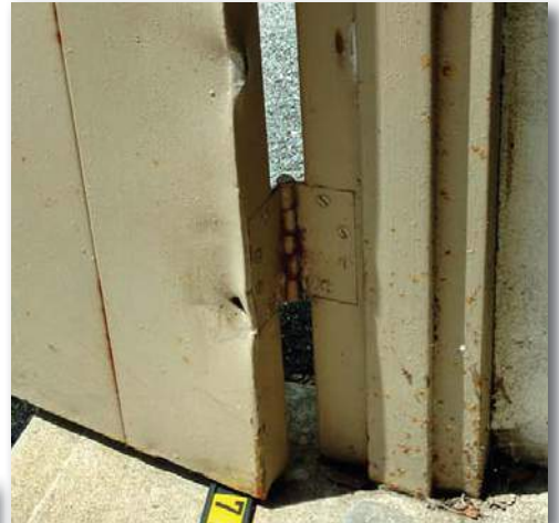
Rusting and rotted door leaf and frame. Non-ADA compliant, damaged door.
