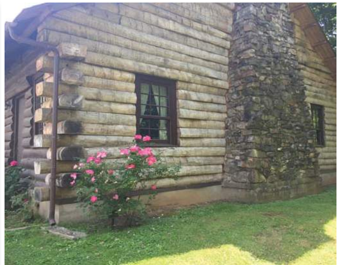
Reconstructed South Facing Side. Drainage Plane still inverted as shown above.
