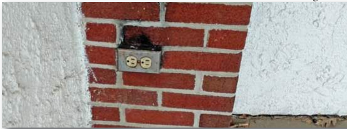
Non-compliant, non-GFCI exterior outlets.
