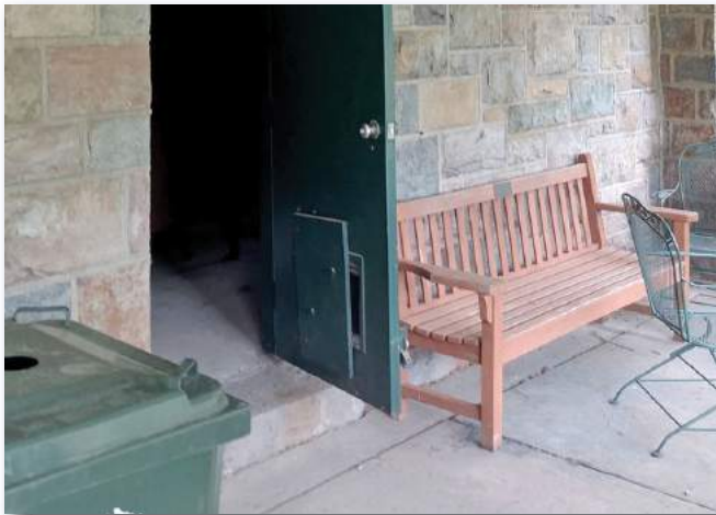
Non-ADA compliant entry way.
