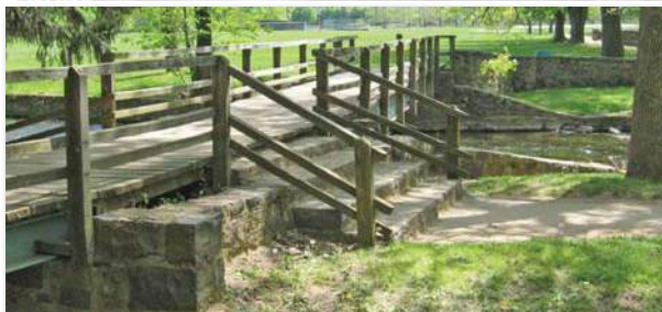
Bridge Crossings and Benches not accessible. Typical.
