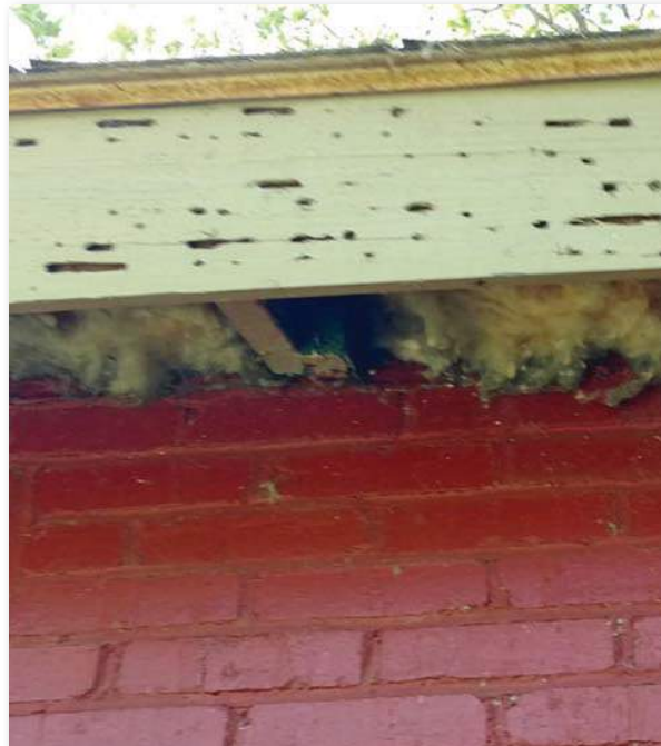
Missing soffit, exposed insulation, and insect damaged fascia board.
