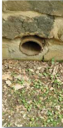
Exposed piping, no insect screens.
