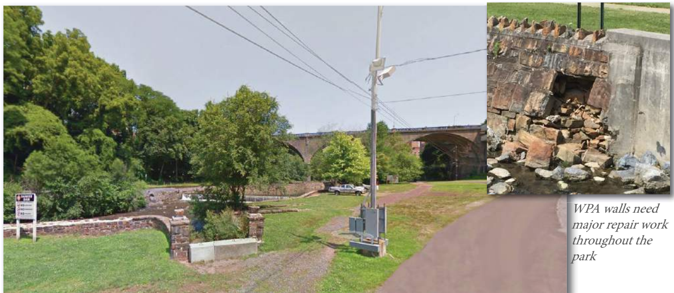
Monocacy Creek lined with WPA walls. Monocacy Way runs adjacent along Old York Road. Riparian restoration and pedestrian gathering spaces would create an engaging park experience.
