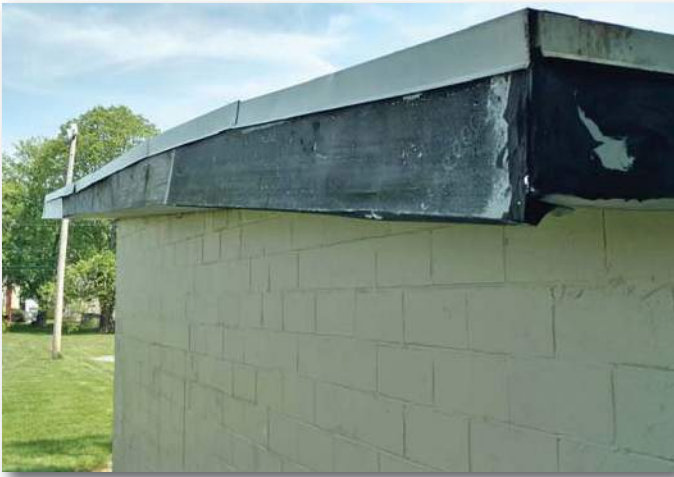
Building #2: Roof sagging and improperly installed coping.
