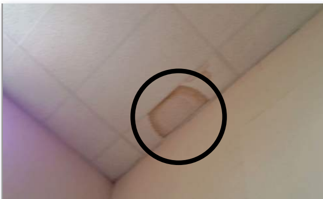
Water damaged ceiling tiles.
