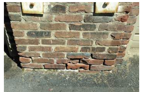
Damaged and degraded masonry and mortar joints.
