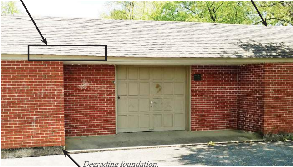
Worn roof edge, rotting frieze board, degraded and missing shingles.
