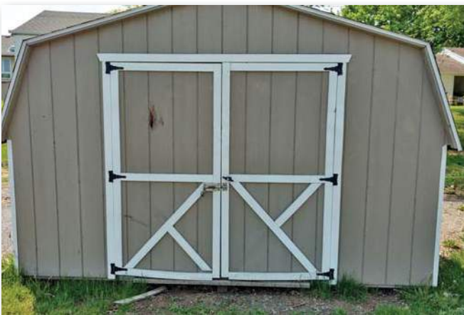
Building #3: Located adjacent to Building #2. Damaged siding.
