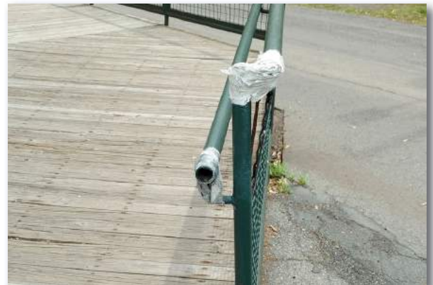
Damaged railing, not ADA compliant as shown.
