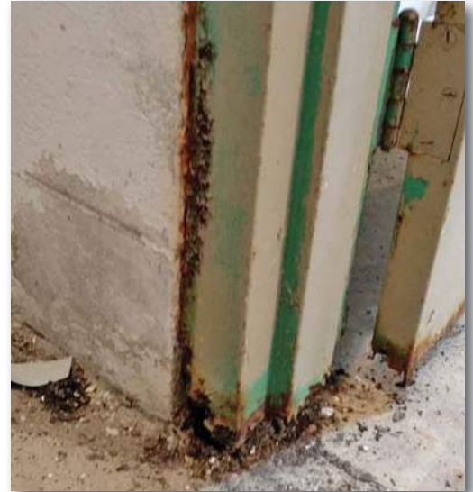
Severe degradation to door frames and doors.
