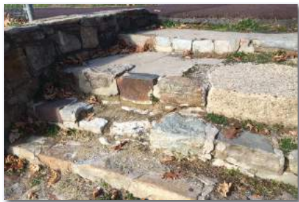
Failing Stone Steps and sidewalks surrounding the park prevent access
