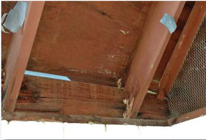
Rotted and damaged structure.
