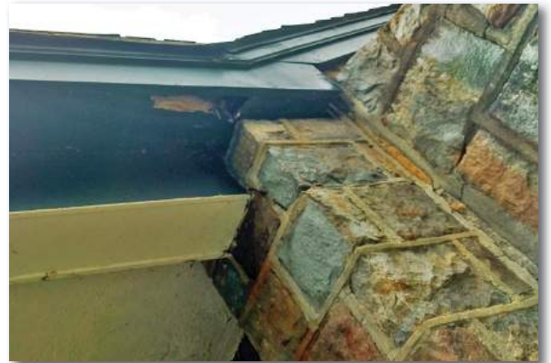
Rotting, holes, and damage to soffit, Typical.
