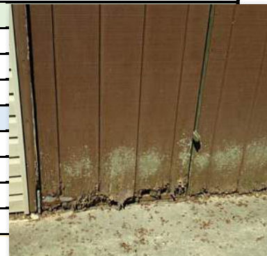
Storage Shed: Rotting doors.
