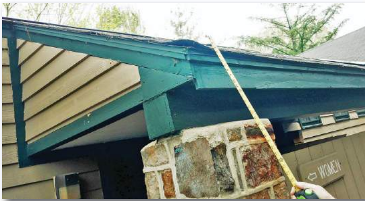
Asphalt shingles are peeling away at roof edge.
