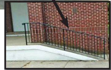
Non-ADA compliant ramp.
