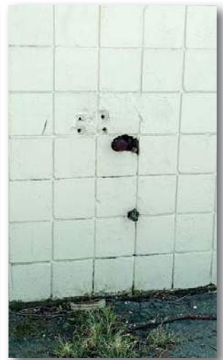
Holes and damage to exterior CMU.
