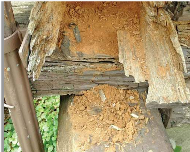
Rotting log construction on multiple sides.
