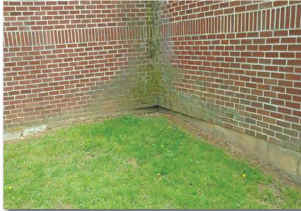
Degrading brick facade and mortar joints due to water infiltration from missing downspouts, typical.
