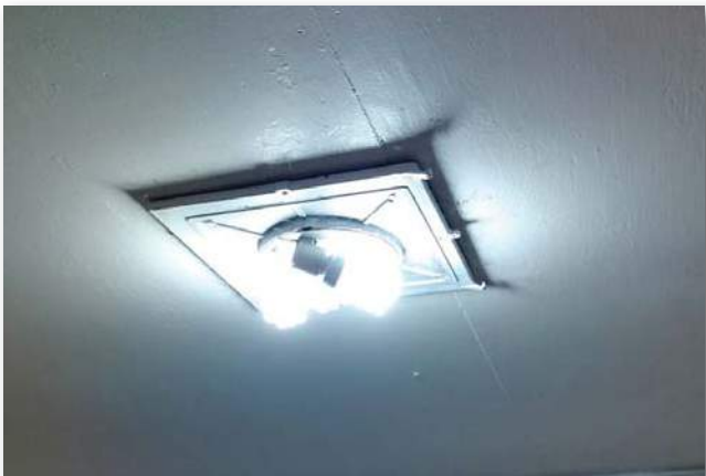
Lighting is missing protective covers, typical.
