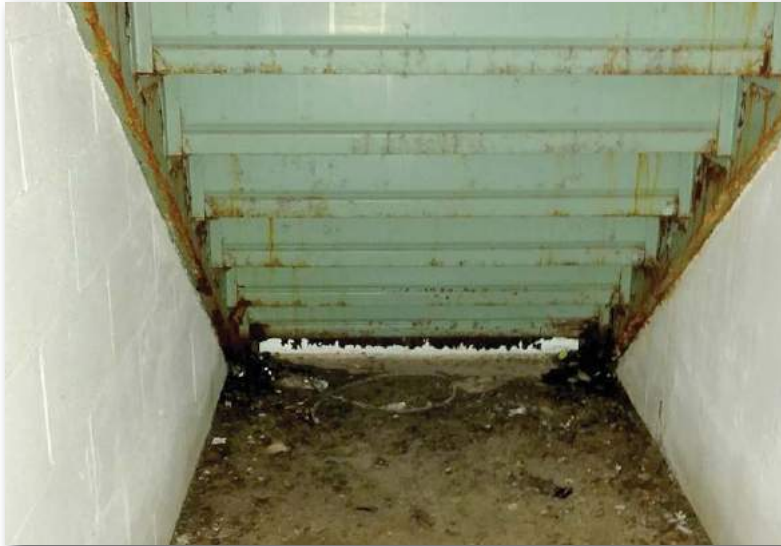
Rusted and rotted stair pans and stringers.
