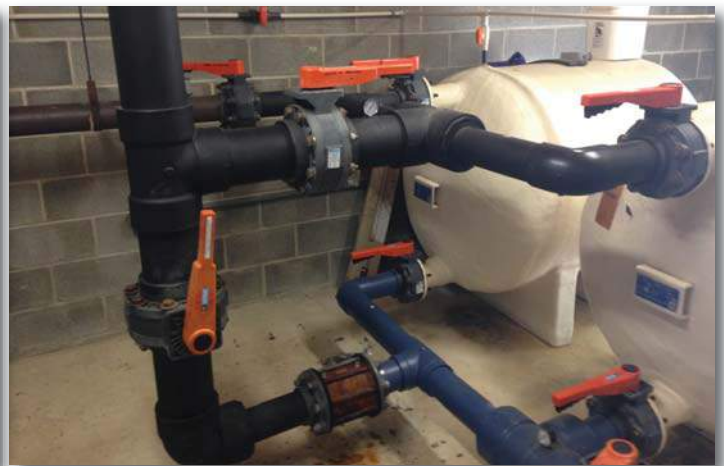
Corroded Flow Control Valve & Filter Tanks - Main Pool
