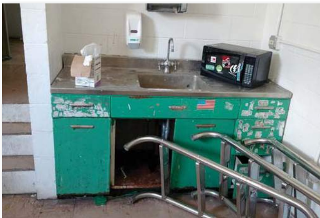
Building interior is in disrepair, typical throughout.
