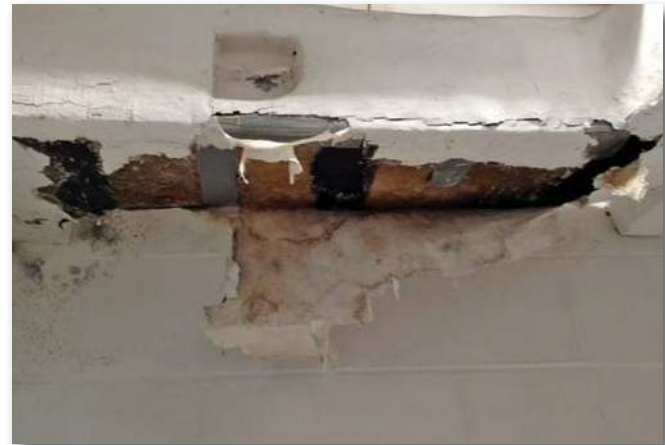
Water damaged insulation on ducts and piping.
