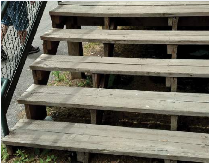
Damaged and worn exterior stair treads and stringers.
