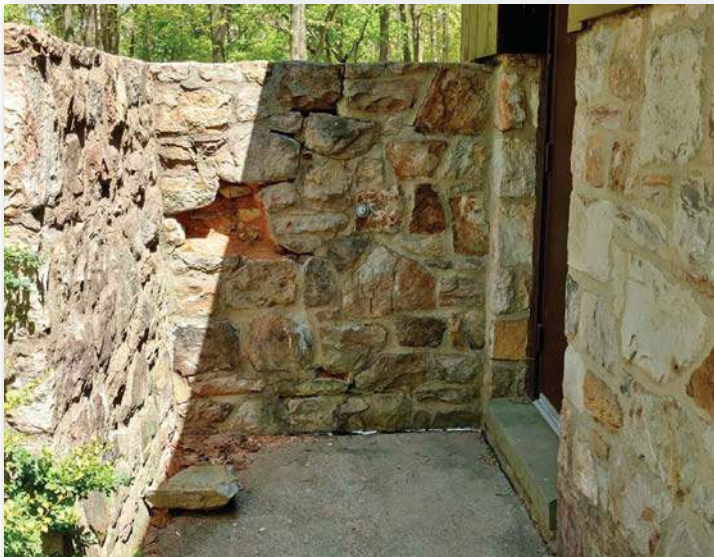
Toilet Room Facility: Degrading pointing and falling stone, typical.
