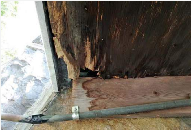
Pavilions #1 and #2: Rotted wood structure and roof decking.
