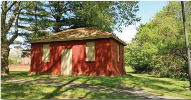
This building is boarded shut and was not available for interior inspection
