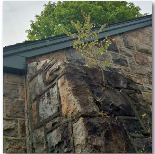
Invasive plants in stonework. Possible areas for future water infiltration.
