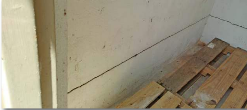
Several large long horizontal cracks, indication of possible structural issues.
