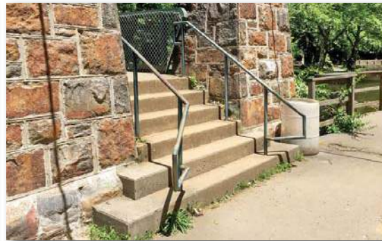
No ADA access for Bridge Crossing
