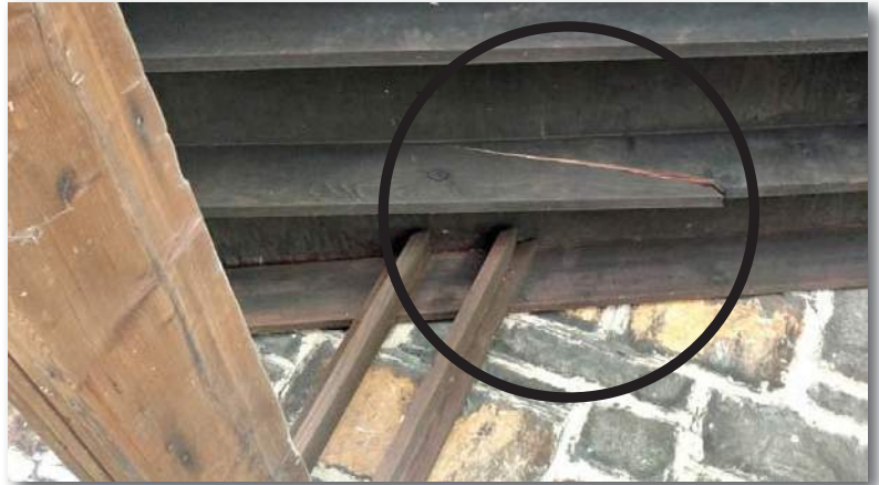
Pavilion #1: Horizontally cracked roof structure.
