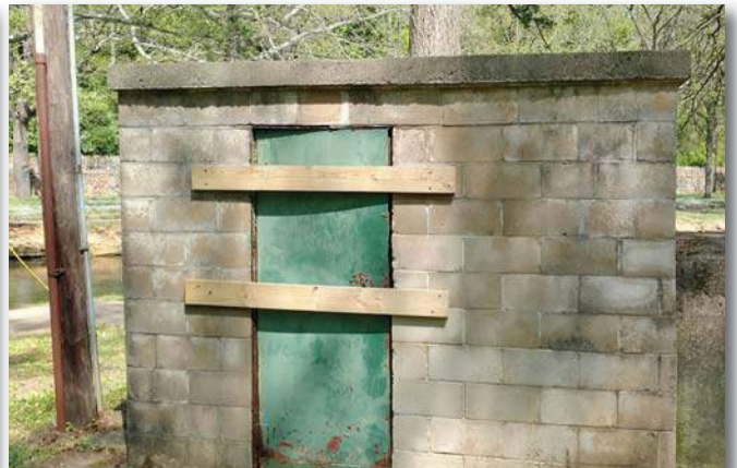
Pump House: Unsafe baring of entry.
