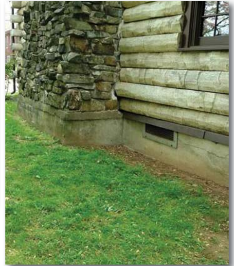
Inverted drainage plane. Typically, missing downspouts.
