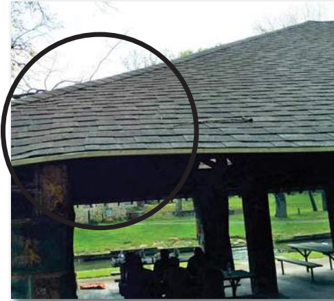
Pavilion #1: Roof is sagging and buckling
