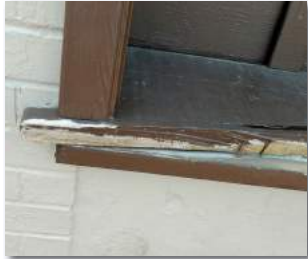
Rotting/damaged concession transaction window counter.
