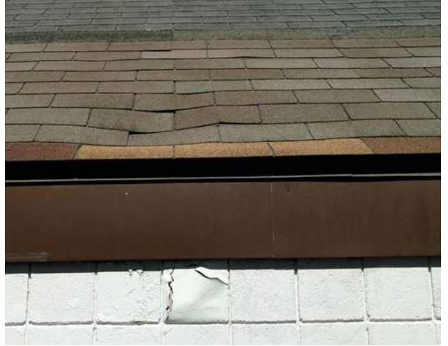
Worn roofing, rotten decking, patched roofing, loose fascia, and loose drip edge.
