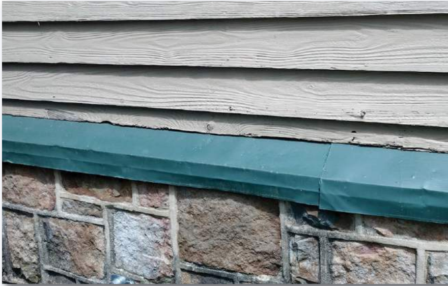
Flashing is damaged. Starter course of siding is rotten. Masonry pointing is missing in places.
