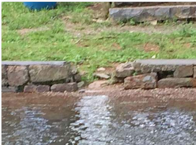
WPA walls lining Saucon Creek crumbling and dangerous. Riparian buffer restoration and limited creek access should be considered. Footpaths degrade soils and vegetation.
