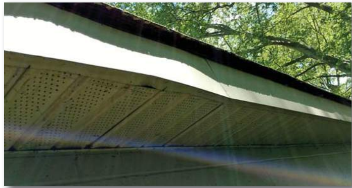
Soffit and fascia board show signs of wear and damage.
