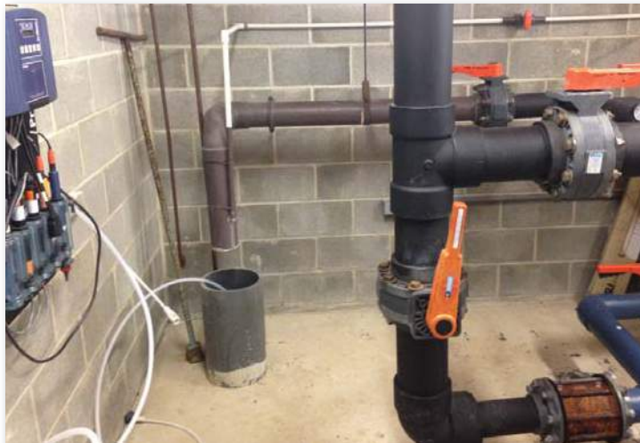
Backwash Line with Air Gap & Chemical Control - Main Pool
