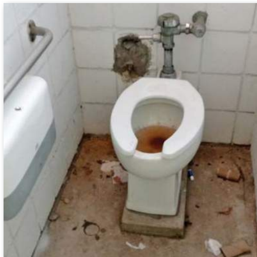
Non-ADA compliant toilet rooms.
