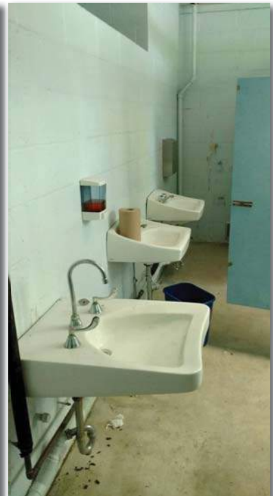
Non-ADA Compliant Restrooms, Facilities and Access
