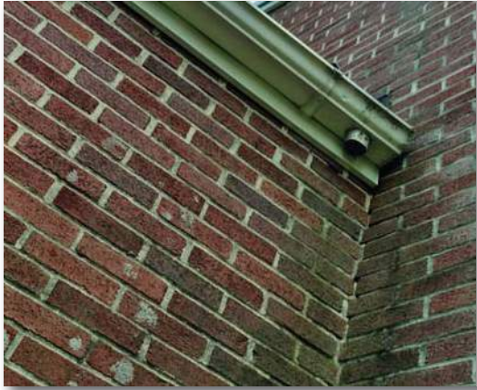
Missing gutters and downspouts, typical.
