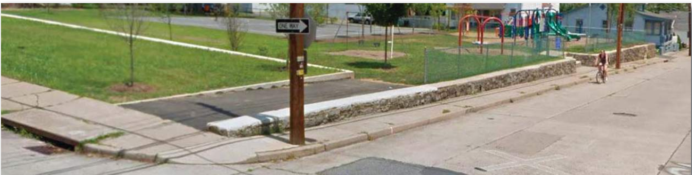
ADA access ramp into Higbee Park. ADA compliant Curb Ramps and Crosswalks missing.
